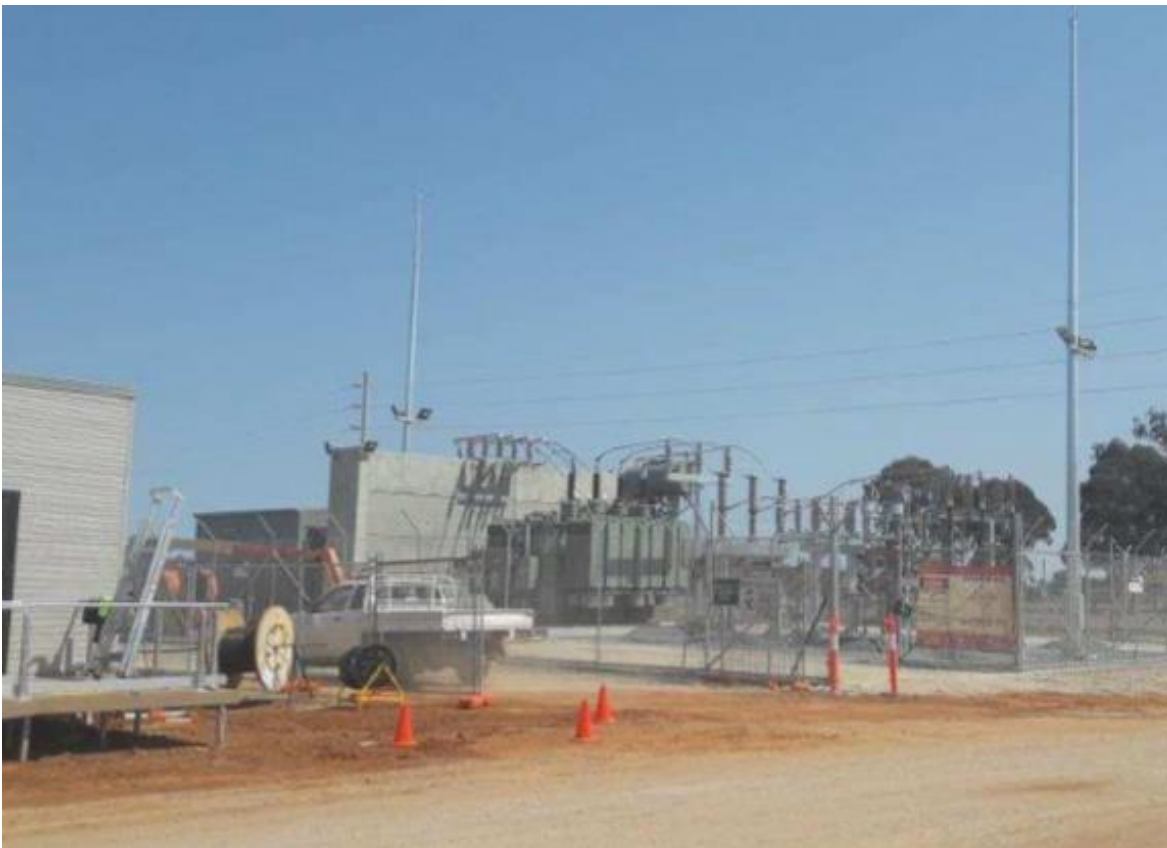
Inverter Station Connection
