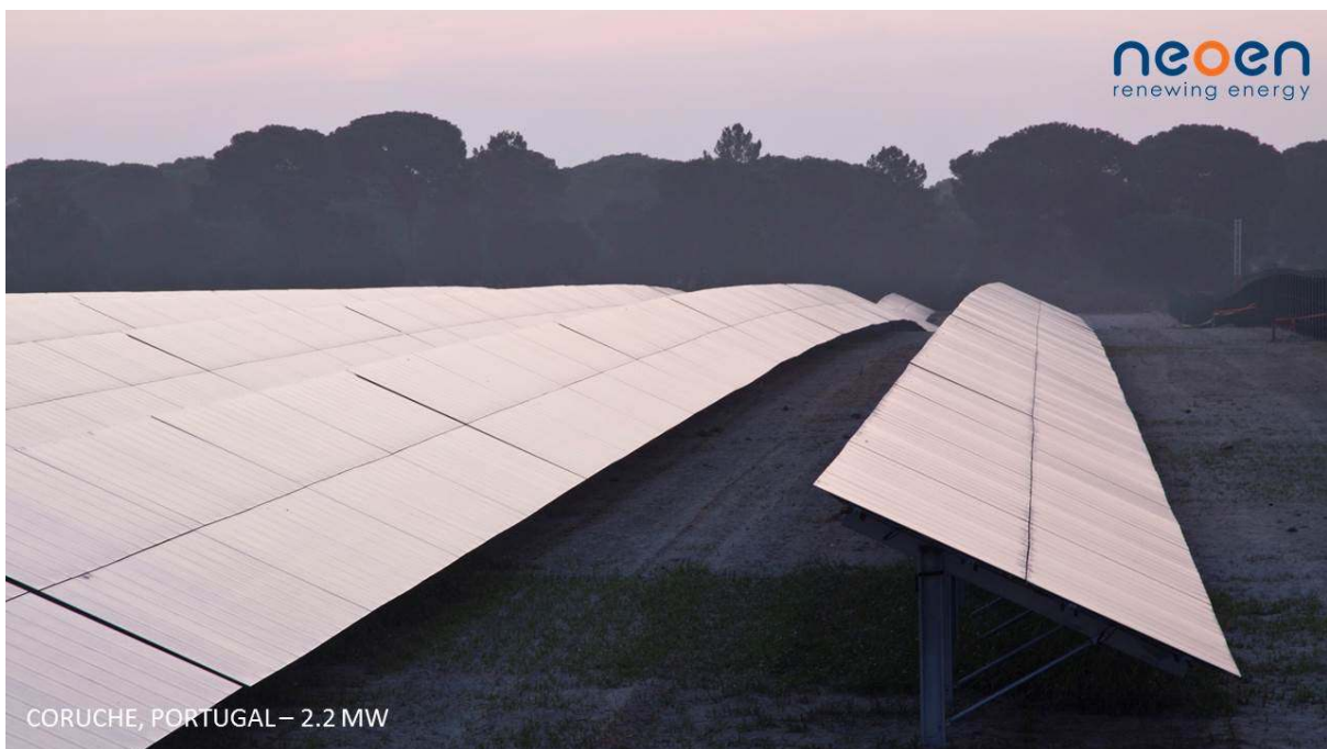
Figure 2-4 Example of south-facing fixed-tilt mounting system with thin-film technology in Europe (installation in Australia would face the north)
