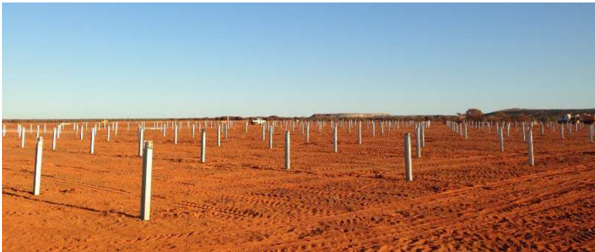
Figure 3-8 Example of poles driven into the ground on a Neoen solar project in Western Australia
